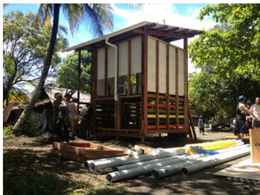
Figure. 4 Three composting toilets were built in Papua New Guinea with students taking more control of the process as the construction phase moved forward.
