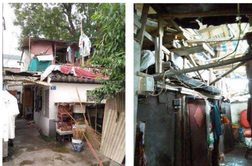
Fig4 the current condition of spontaneous reconstruction on site (Source: photographed by author)
