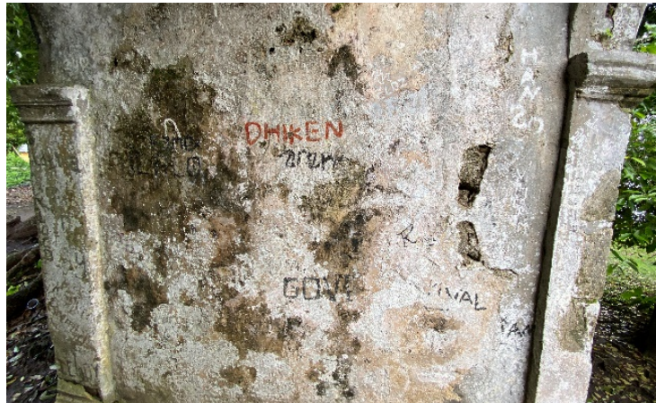
Figure 3: The Condition of the Walls of Fort Hollandia Where Many Graffiti Were Found
