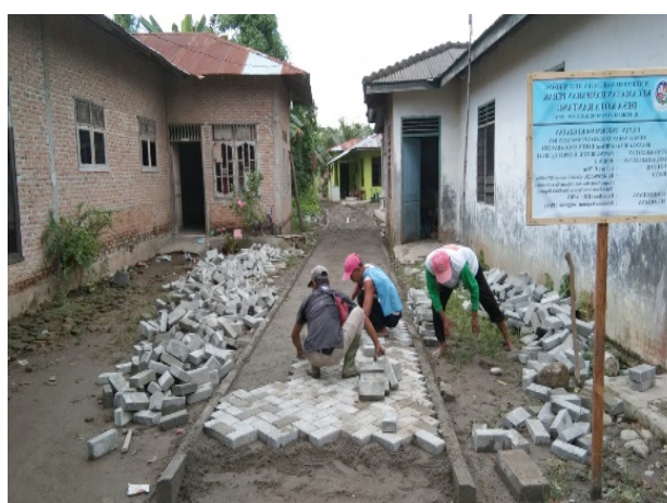
Figure 2: The process of installing paving blocks for the people of Rantang City Village
