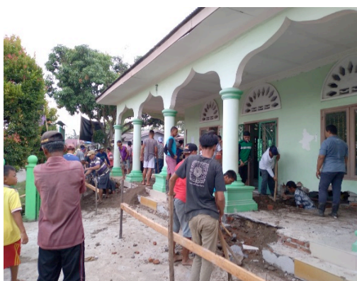
Figure 1: The process of building a mosque with the people of Kota Rantang Village
