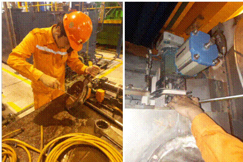
Figure 5. Activity of Re-Design Waste-Gate Valve: (left) Dismantling the Waste-Gate Valve in PLTDG 10 Pesanggaran; (right) Assesmbly the Re-Designed Waste-Gate Valve in PLTDG 10 Pesanggaran.
