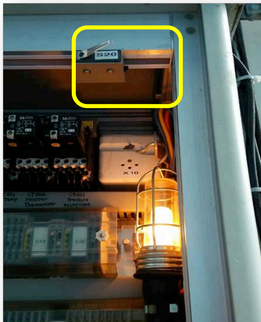
Figure 3. One of Motion Detection System in Gilimanuk GTPP
