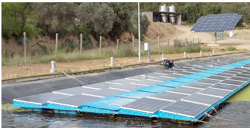
Figure 1 Floating photovoltaic set and solar tracker photovoltaic set
