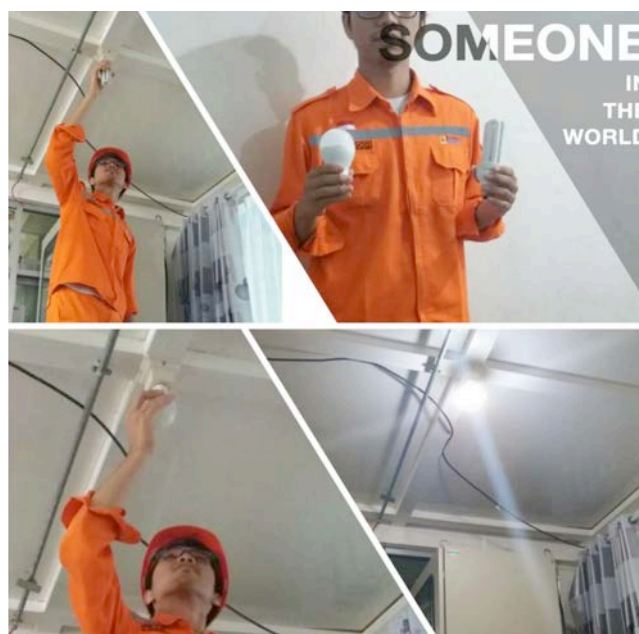
Figure 5. Substitution of Mercury Lamp to LED in Office Building
