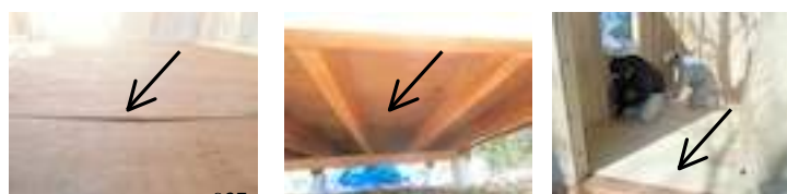
Fig.3-2 Broken part and solution
